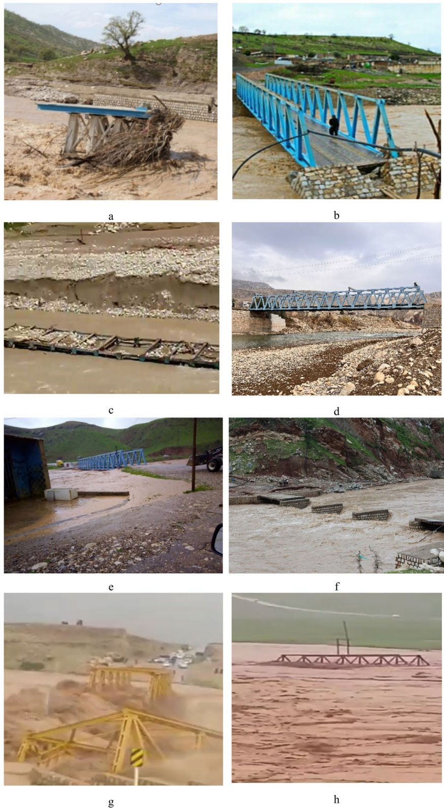
Fig. 5 Post-flood conditions of the investigated steel truss bridges: a collapsed STB1, b STB2 collapsed due to abutment scour, c STB3 after the flood, d STB4 after the flood, e STB5 during flooding, f collapsed STB6, g STB7 during flooding, and h STB8 during flooding
